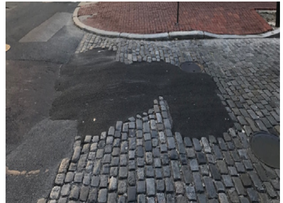
After an email to our contact at the Streets Department, the pothole was patched. Not a pretty sight, but they will return in the spring to repair it properly.
